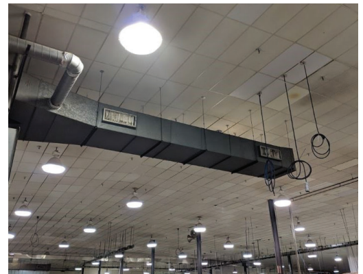
LED lighting at Elmer Candy facility.
